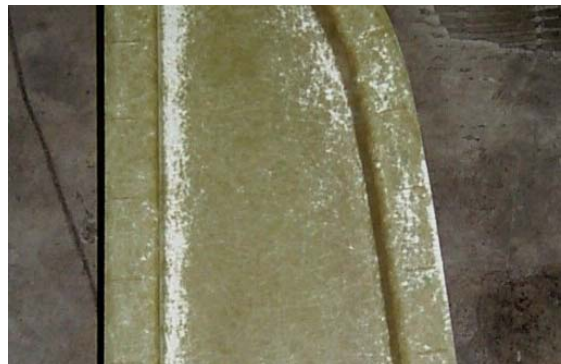
Figure 7. Areal density distribution issues in a molded B-pillar outer, 1.5 mm section, glass fiber preform
